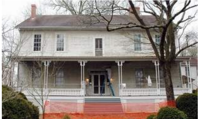
Workers from the Alabama Correctional Industries make renovations to Gen. Joseph Wheeler's home at Pond Spring, near Courtland. (Deangelo McDaniel)
